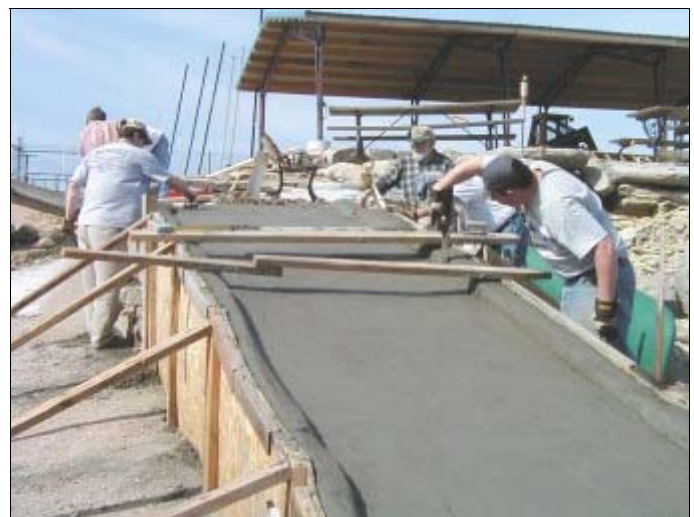
Putting the finishing touches on the sloped ramp between the stone jetty and water's edge on March 15.
