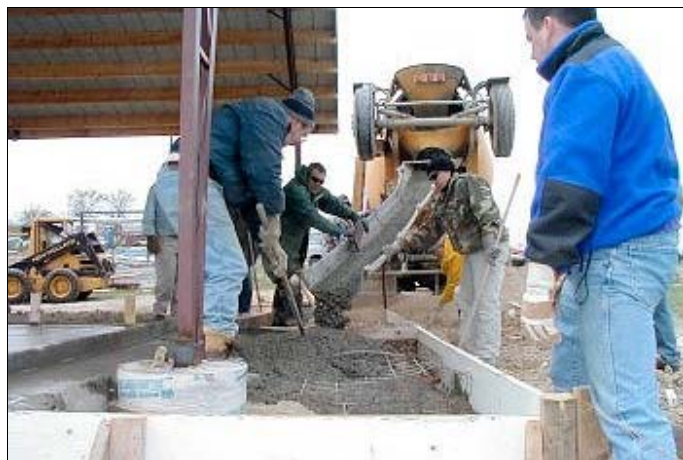
Guiding the flow of wet cement from the ready-mix truck and spreading it over the reinforcing mesh wire
