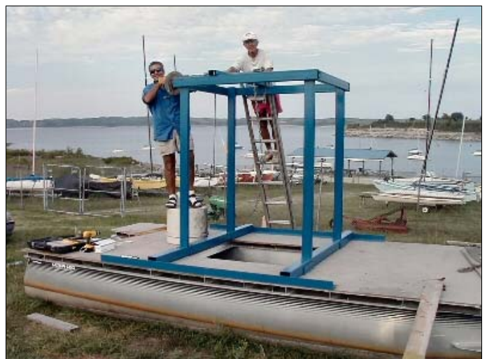
Wayne Martin and Bob Mullen Installing bomb winch on new work barge
